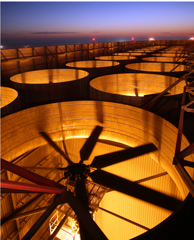
Cooling towers located at industrial facilities.
